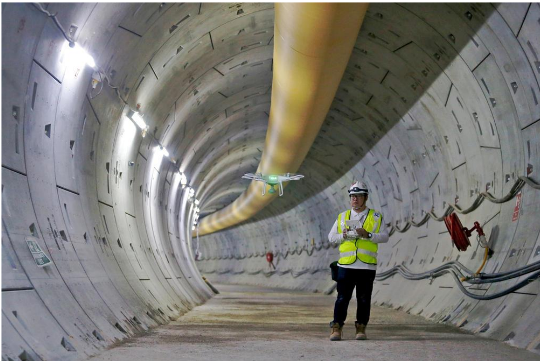
Figure 6: Inspection in the TEL Tunnel between Orchard and Orchard Boulevard stations Source: TODAY, 2017
